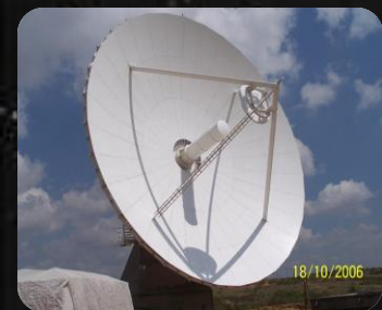
18m Terminal -operational
