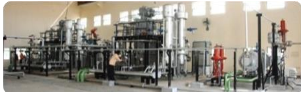
Hypersonic Wind Tunnel Test Facility
